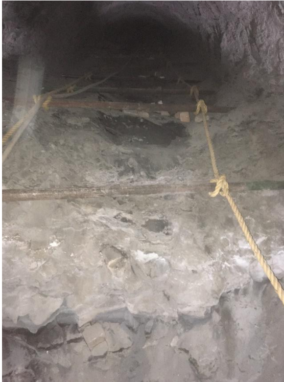
Damaged and fine clinker dust in TAD
