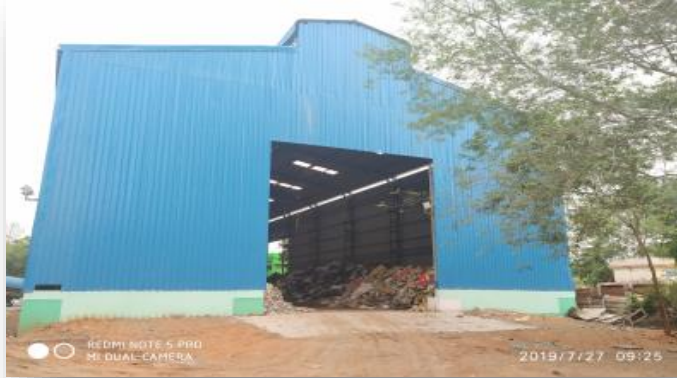
1. Shredded material Storage Shed
